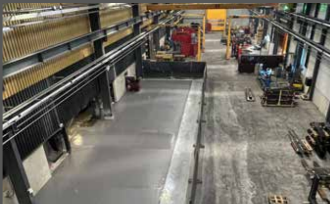
The metalwork area is progressively taking shape. Recently, tailor-made flooring was put in place for the future boring machine, which will be delivered in the next few months.
